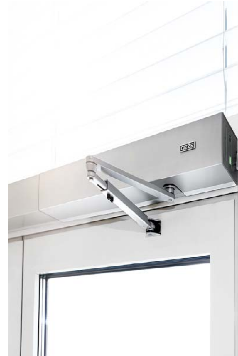
Automatic Swing doors
